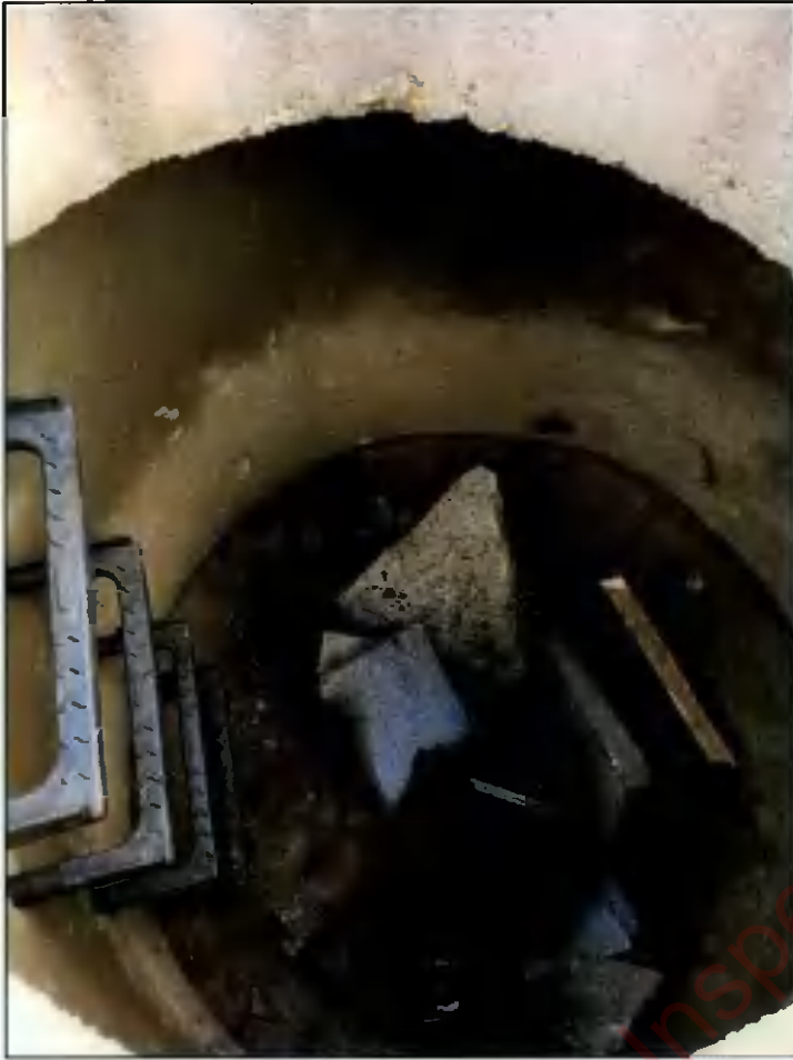
Plate 3-5. Open manhole located west of surface water feature. It should be noted the flow of water was in a westerly direction into the water feature.
